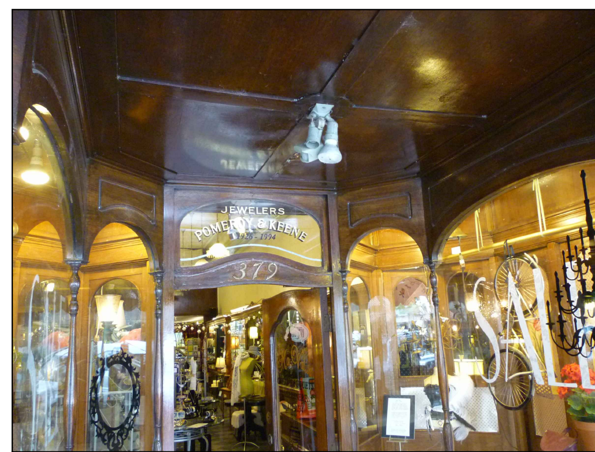
D. MA VALISE ENTRANCE; EXISTING WOOD PANELING AND TRIM TO BE REFINISHED. LIGHT FIXTURE TO BE REMOVED AND REPLACED
