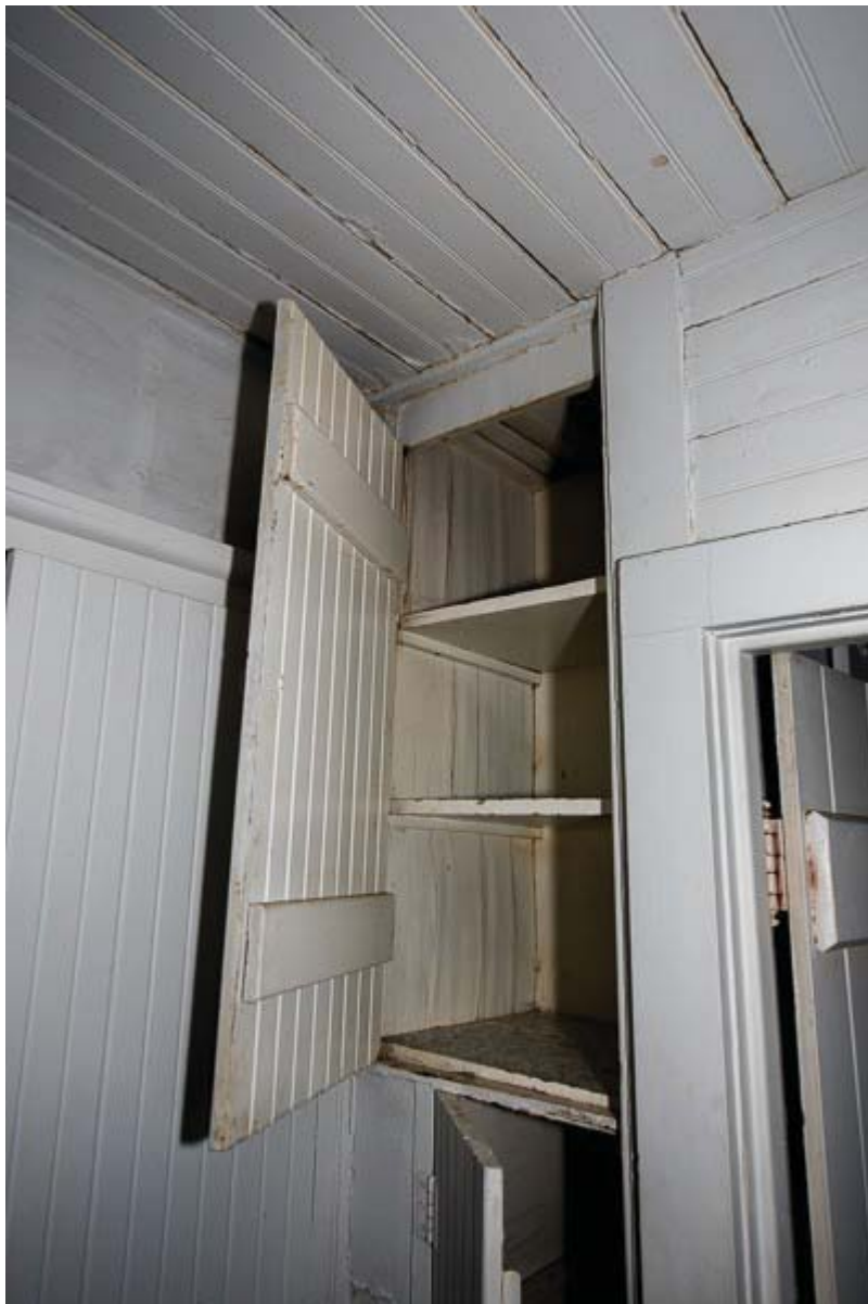
Figure 19: Water Damage Next To Chimney In Kitchen
