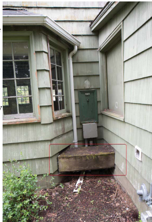
Figure 16: Exterior Heating Duct Serving Bay Window
