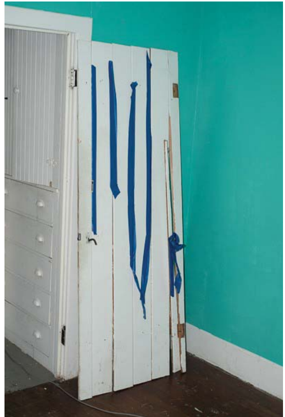
Figure 3: Smashed Interior Door from Tenant Rampage
