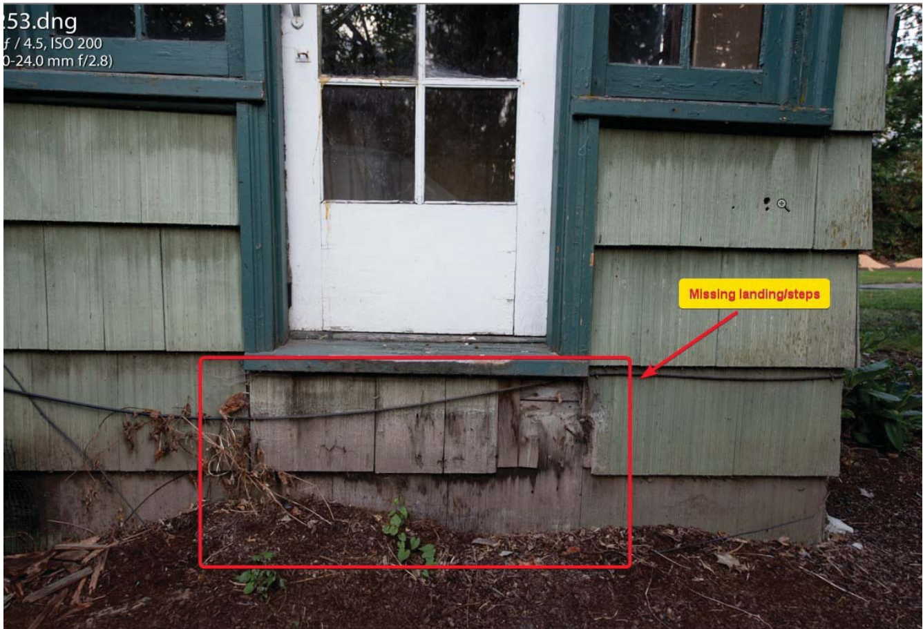
Figure 13: Eastern Facade Showing Missing Landing
