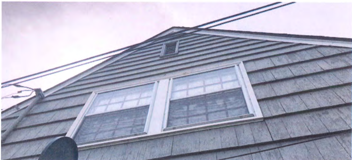
East Façade – 2 nd Floor- Window 8, 9
