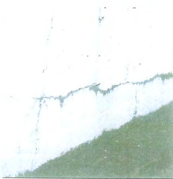
5. Crack in Ramp Wall
