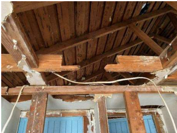
Photo 11: Cut Ceiling Joist
