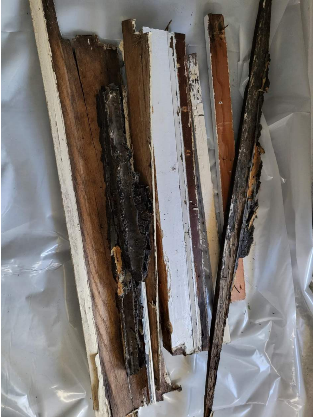
Existing sash and trim in poor condition
