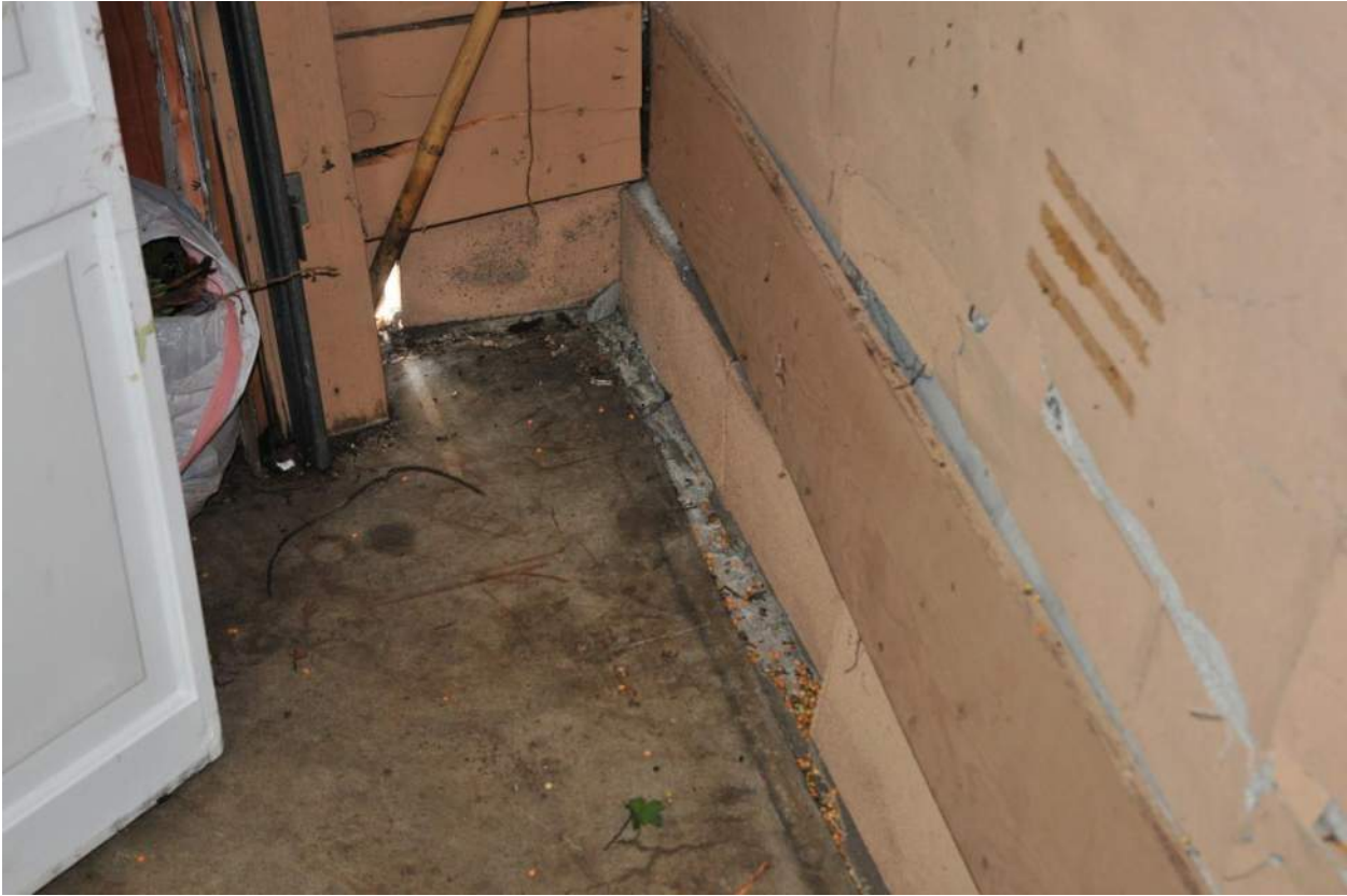
Block wall shifted:
