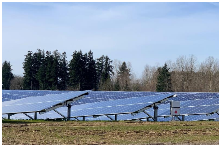
This Keizer-area solar array's capacity is just under 1 MW.
