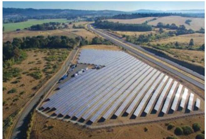
This nearly 3-MW solar array outside Willamina launched Portland General Electric's Green Future Solar Program in 2016. PGE customers could "buy" 1-kW blocks of solar.
