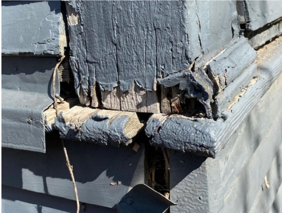
Photo # 7: Existing Condition – detail of corner post (base)- rear porch (southeast corner)
