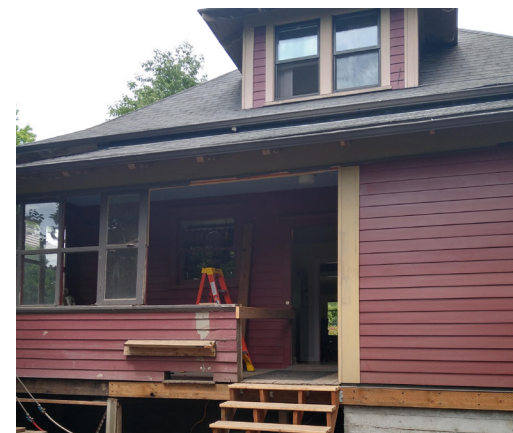
HALF WALL AND MATCHING SIDING AND SILL BEFORE REMOVED DUE TO ROT
