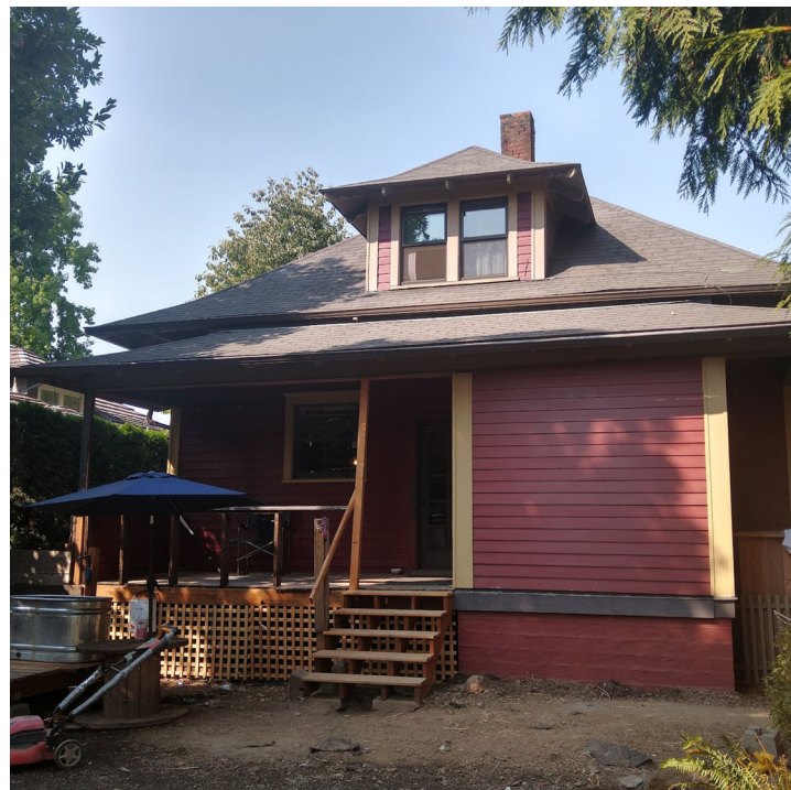
ROT REMOVED, CURRENT STATE, READY TO REPAIR
