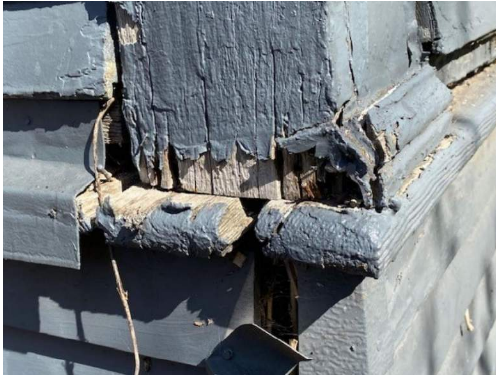
Photo # 7: Existing Condition – detail of corner post (base)- rear porch (southeast corner)
