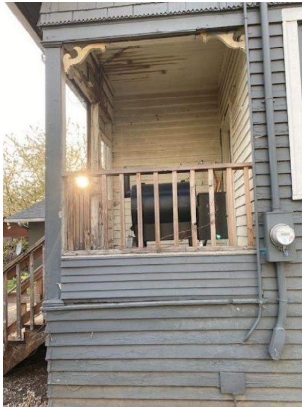
Photo #6: Existing Condition – Detail of porch -rear southeast corner of Hewitt House – looking west
