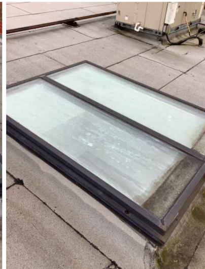
Skylight Seal(s) Failed - Roof (Close-Up)
