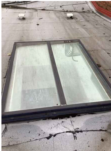
Skylight Seal(s) Failed - Roof (Close-Up)
