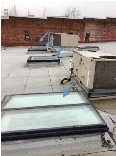
Skylight Seals Failed - Roof
