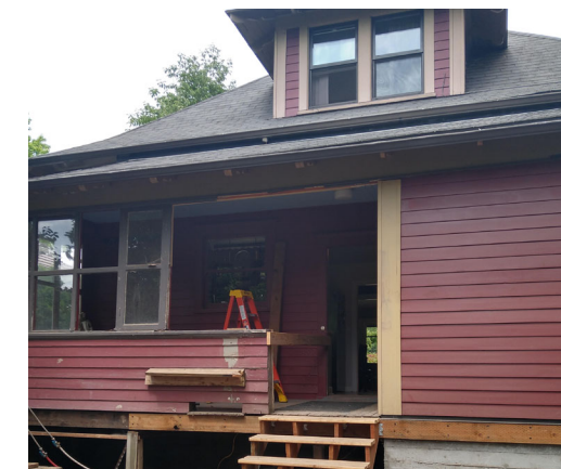
HALF WALL AND MATCHING SIDING AND SILL BEFORE REMOVED DUE TO ROT
