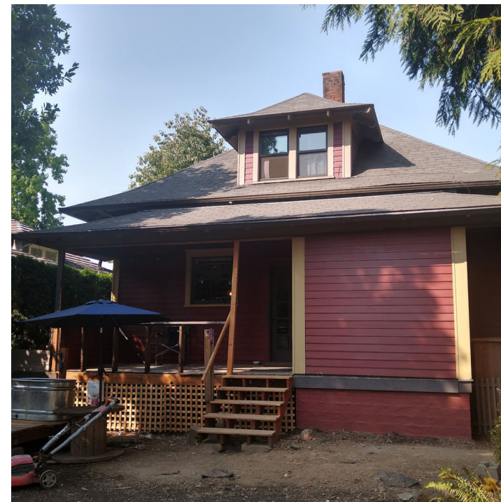
ROT REMOVED, CURRENT STATE, READY TO REPAIR
