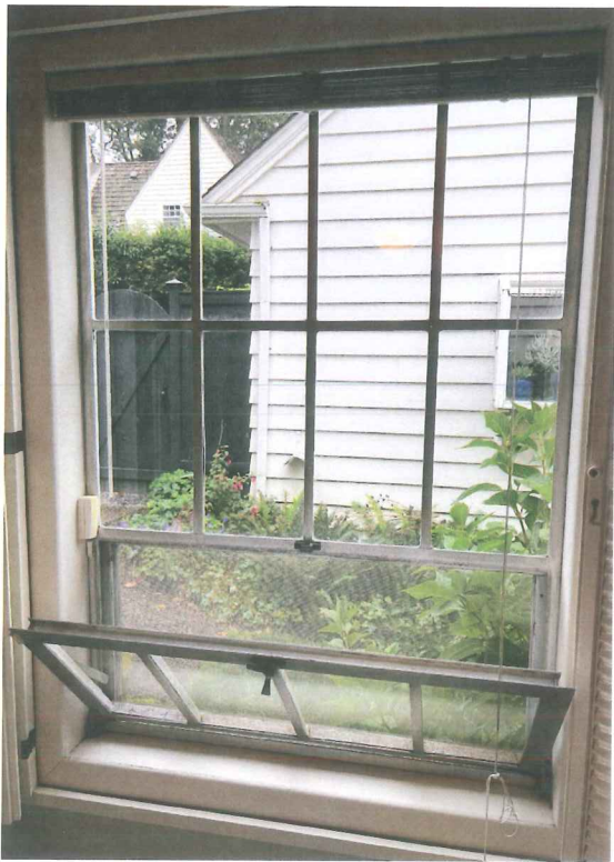
Figure 4 – Photo of east bedroom window opening from interior showing open hopper transom
