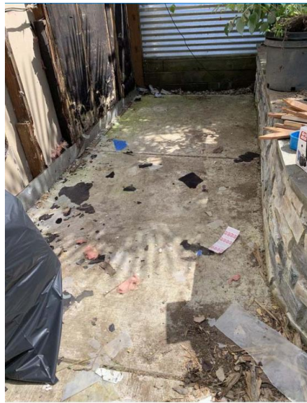
Before Addition – Rotten framing
