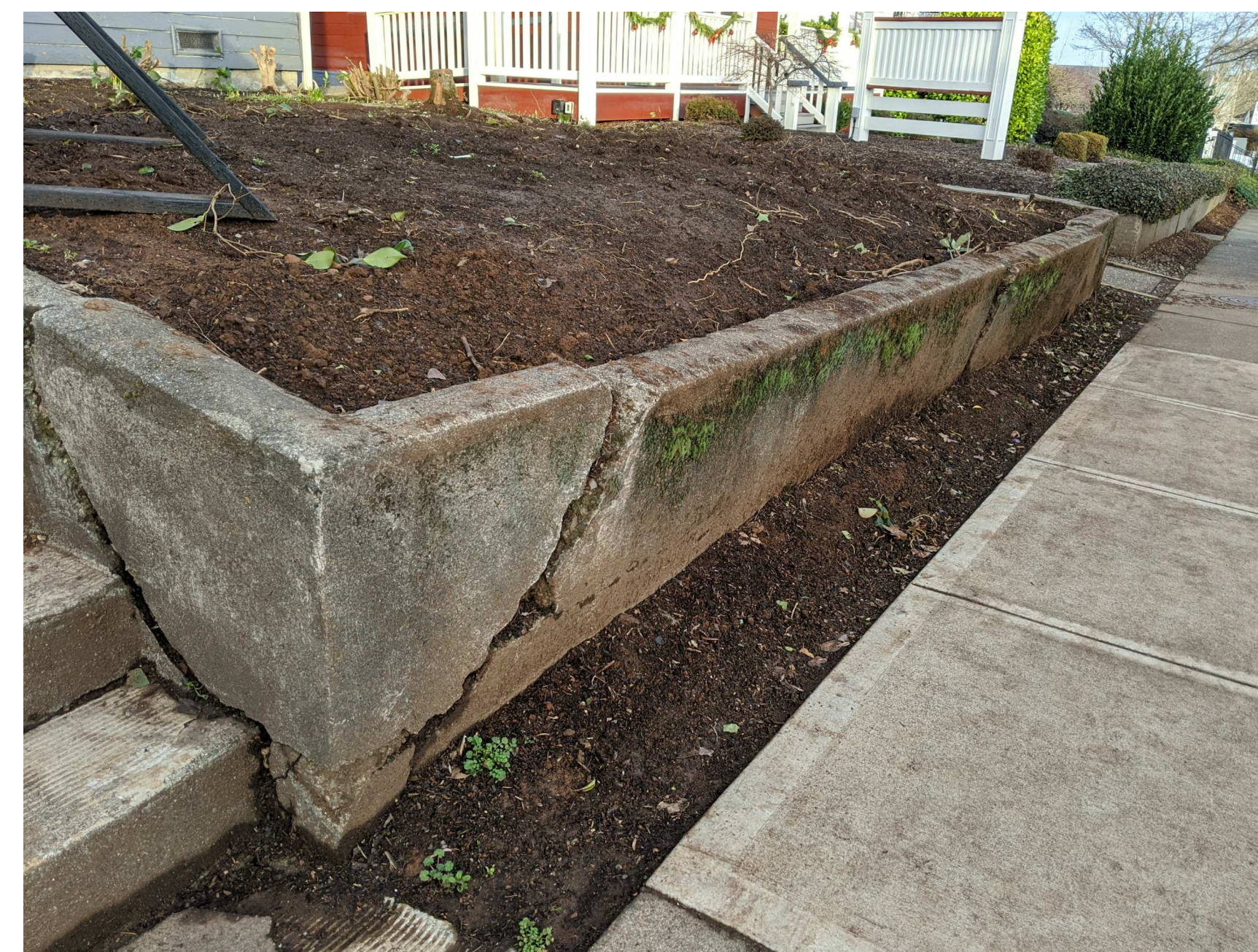
DAMAGED RETAINING WALL
