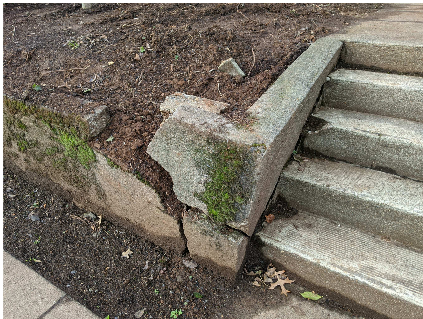
DAMAGED RETAINING WALL
