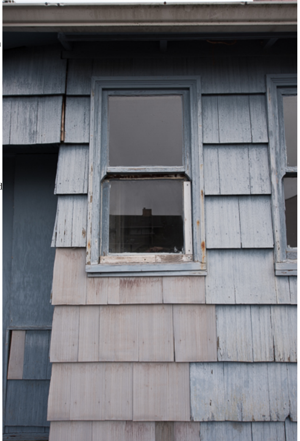
Figure 1: West Kitchen Window 4/3/2020
