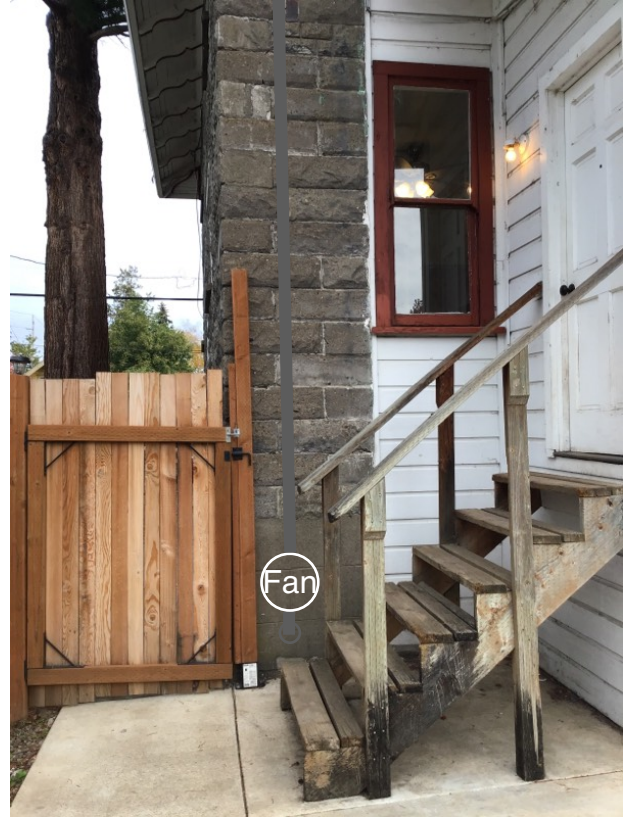
Fan location on rear exterior of home, core drill through foundation stones
