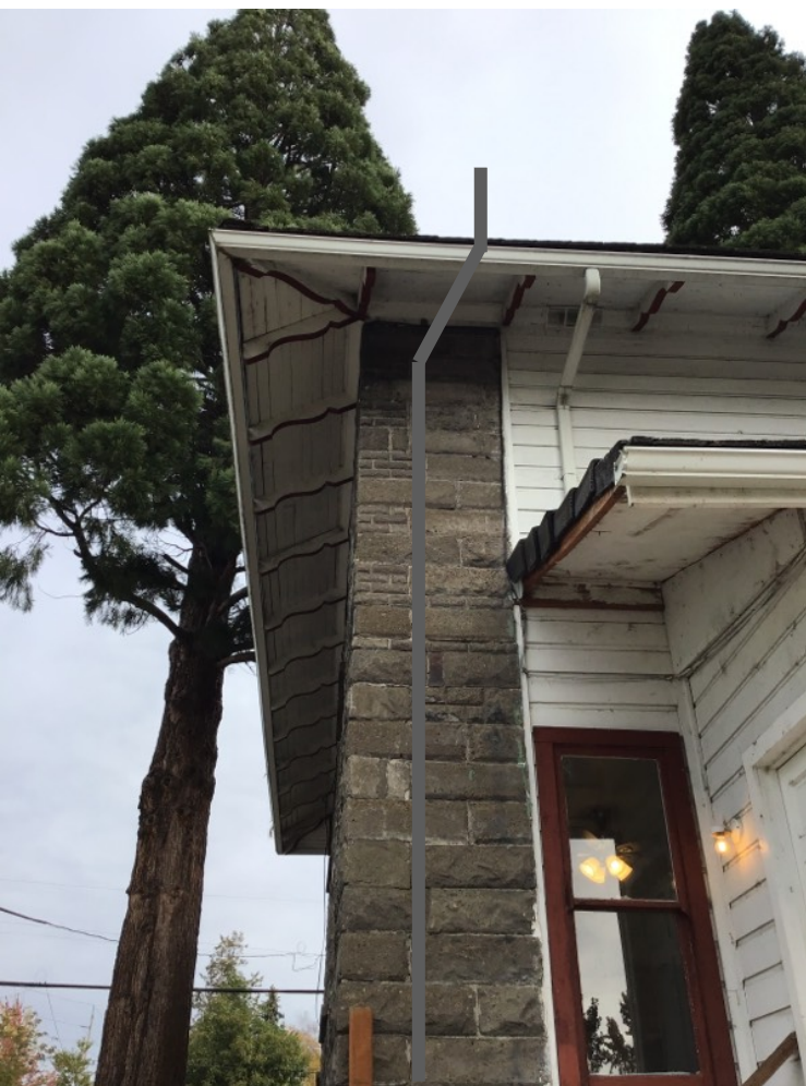
Vent location, pipe routed around rear eave to avoid roof penetration
