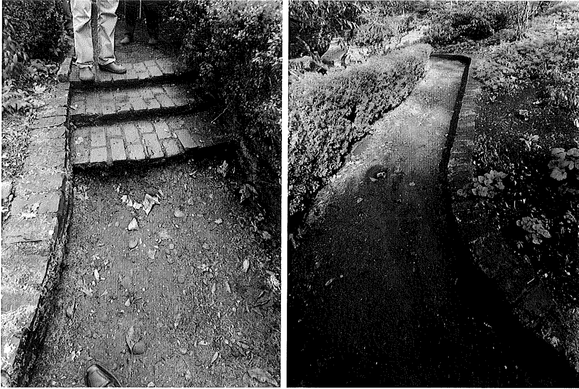
Note the washed out path in the center due to inporper drainage.
