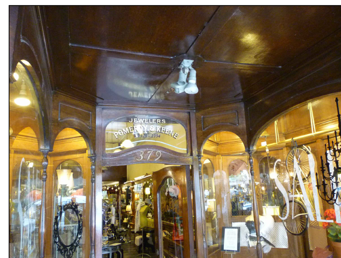
D. MA VALISE ENTRANCE; EXISTING WOOD PANELING AND TRIM TO BE REFINISHED. LIGHT FIXTURE TO BE REMOVED AND REPLACED
