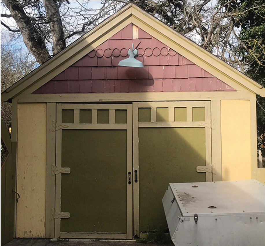
SHOWING PREVIOUS GARAGE DOORS NOW REMOVED DUE TO FAILING MATERIALS
