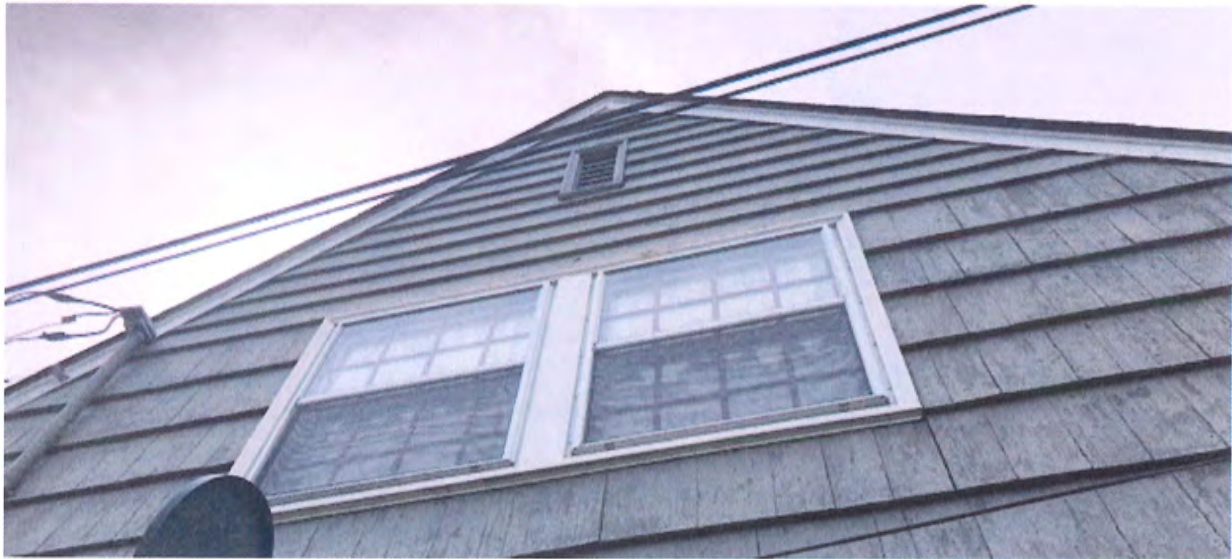
East Façade – 2 nd Floor- Window 8, 9
