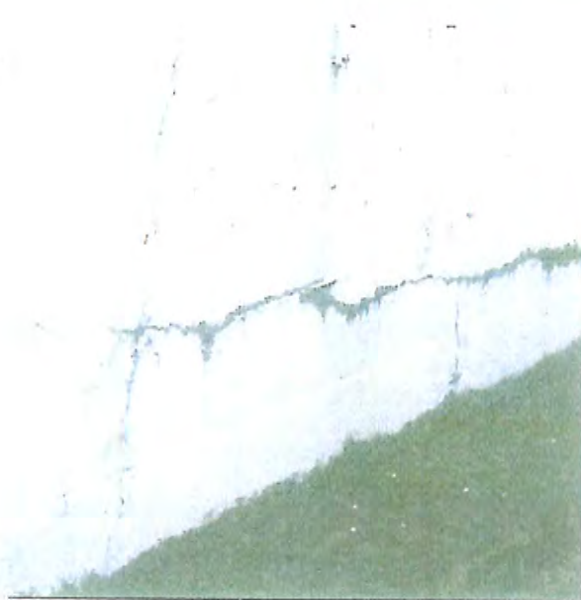
5. Crack in Ramp Wall
