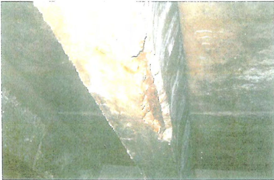
2. Rusting Rebar in Bottom of Concrete Joist
