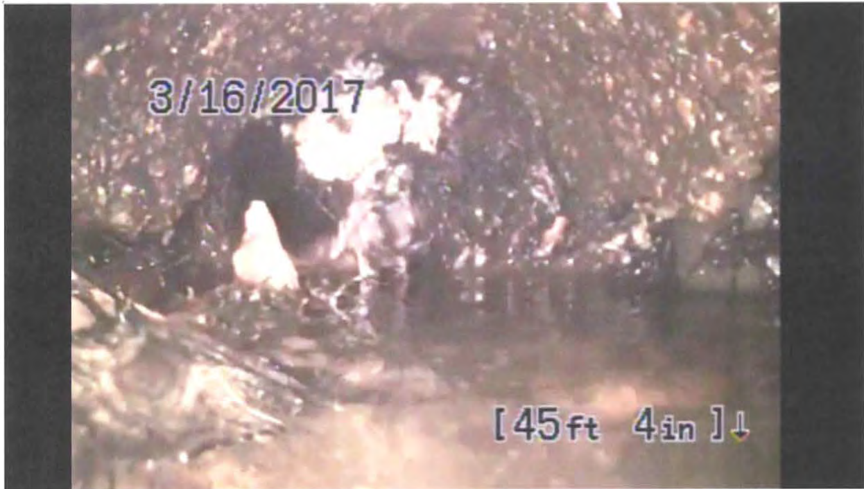
Failed Sewer line
