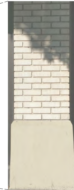
CONCRETE AT PILASTER BASE. COLUMN AT CORNER TO BE RESTORED TO MATCH.
