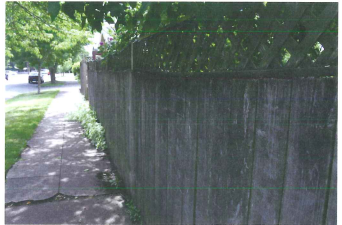
Fence is uneven and many posts have rotted through
