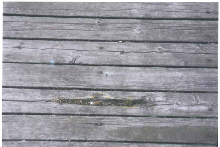
Well-worn stairs (left) and rot in deck boards (top)
