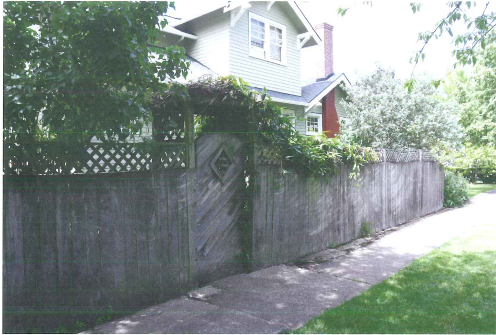
Existing fence - This structure fell during a storm in November 2014. Currently being held up by beams (see below left)
